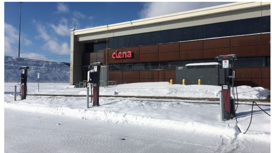
Ciena's EV chargers at offices in Quebec City, Canada
