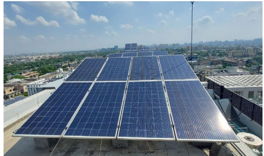
Ciena's PV plant at offices in Gurugram, India
